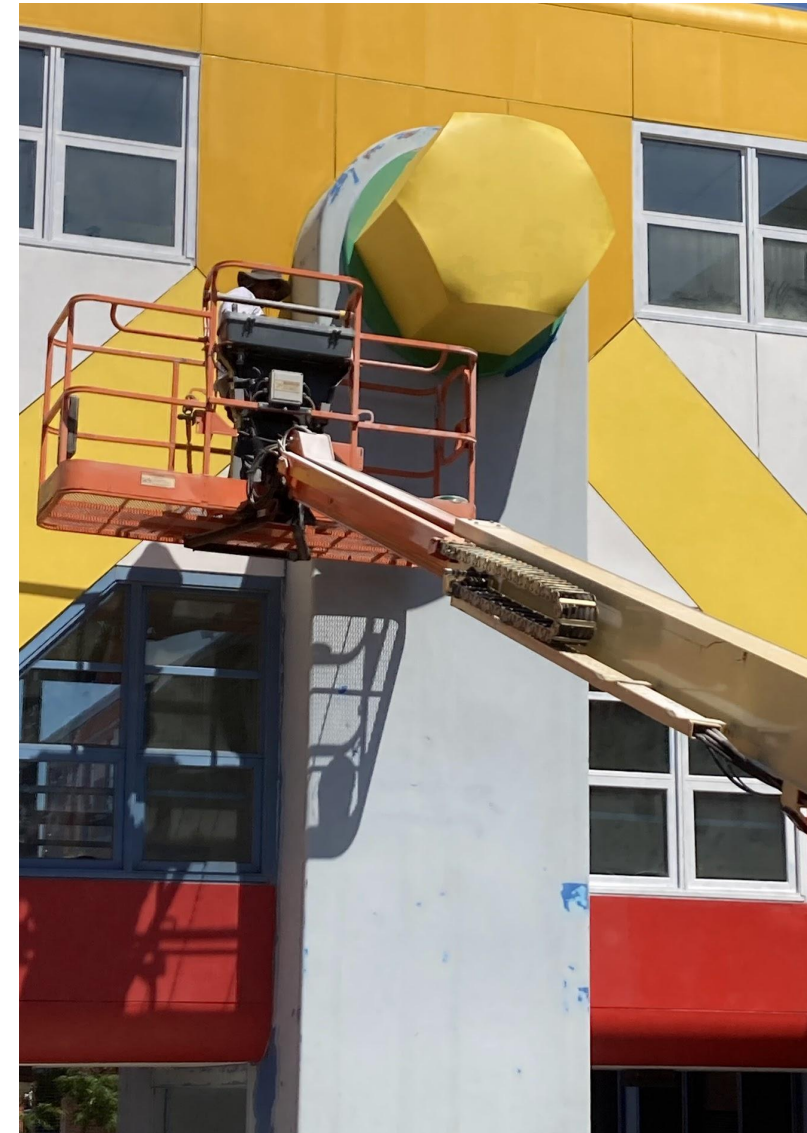
Repainting of Art Benson's "Nut & Bolt" at Mt. Royal Elementary Middle
